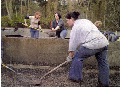
Future home owners working on a foundation -part of the Kitsap Housing Authority project.
